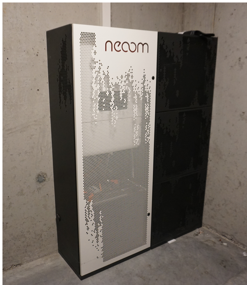
Figure 4.2: BESS installed at LiLa site Source: Vlotte
