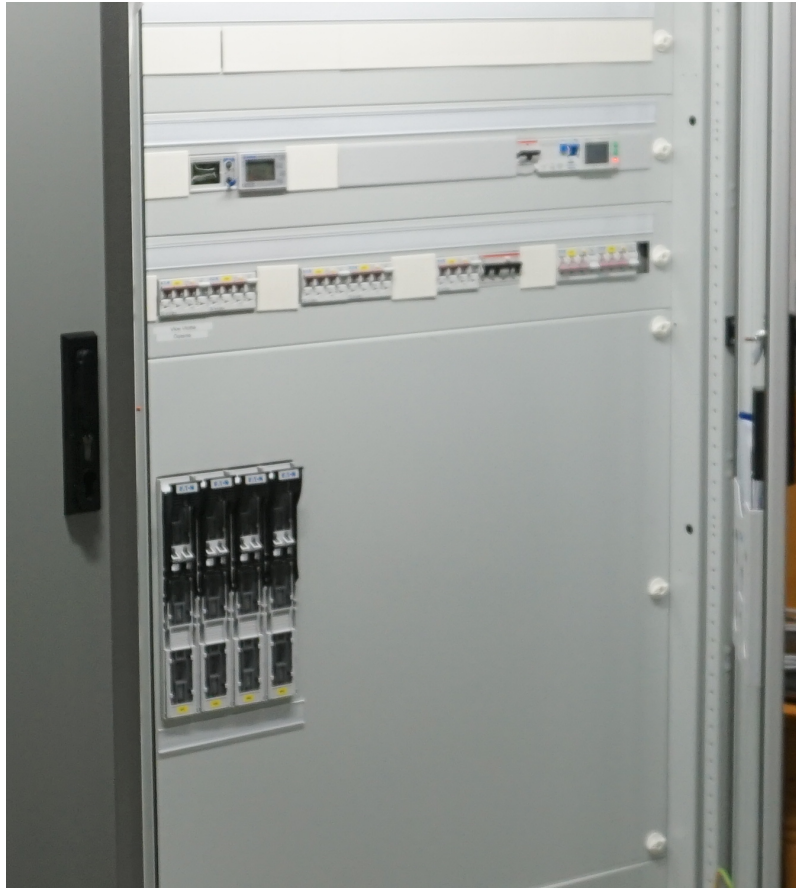
Figure 4.4: Power cabinet installed at LiLa site Source: Vlotte
