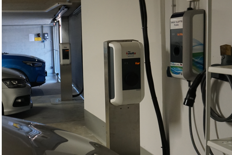
Figure 4.3: Wallboxes installed at LiLa site Source: Vlotte
