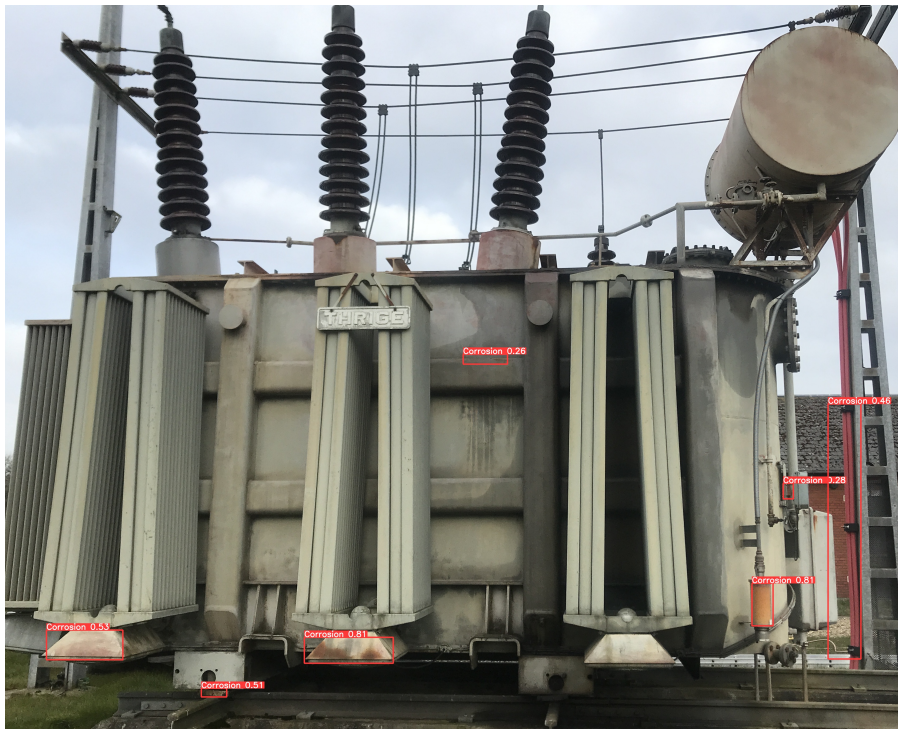
Figure 4.14: Rust Detection on Power Transformer
